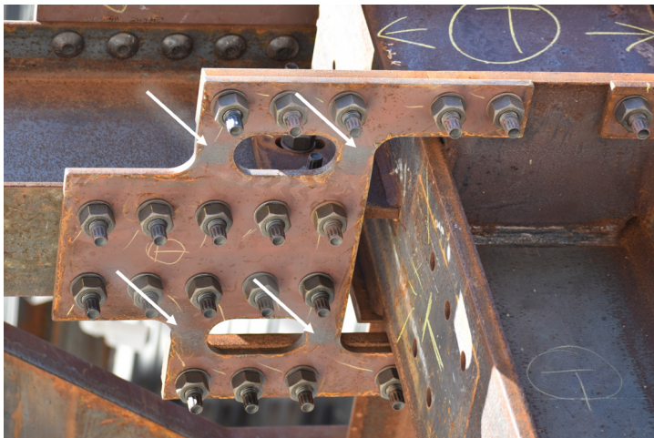
Fig. 3 Mill scale flaking consistent with about 2% story drift.
