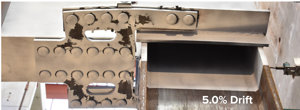
Fig. 2 Mill scale flaking corresponding to different levels of story drift (Richards 2022).
