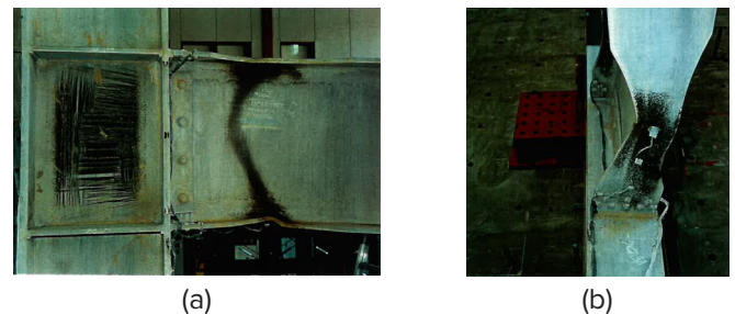
Fig. 4 Results from experimental testing of RBS connection with W36×150 beam: (a) 3% drift; (b) 4% drift (Gilton, Chi, and Uang, 2000)
